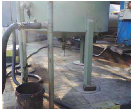
Gambar 5. Kondisi Saddle & Support HSD Tank
